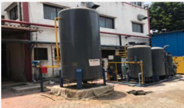
Nitrogen to Oxygen plant by M/s. UPL Ltd. at LG Rotary Hospital, Vapi, Gujarat
