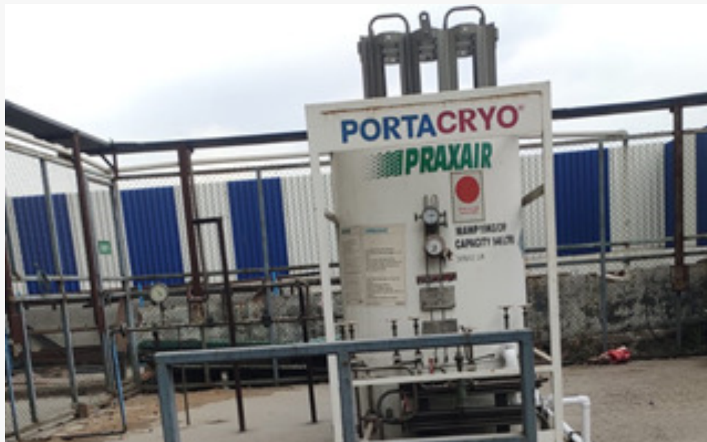
Ultra high purity n2 gas for degassing from inhouse liquid N2 gas plant
