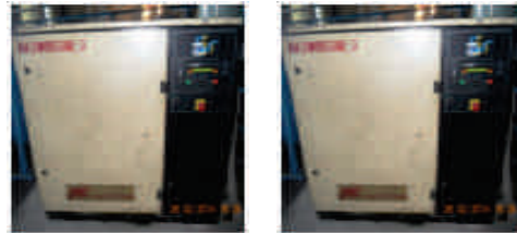
Machines running with 2 compressors 25HP each
