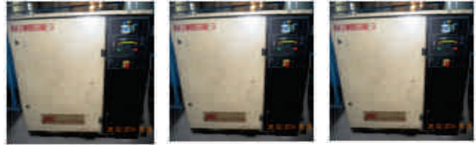
Machines running with 3 compressors 25 HP each
